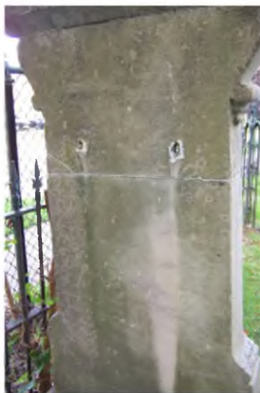
repairs visible on back of marker
